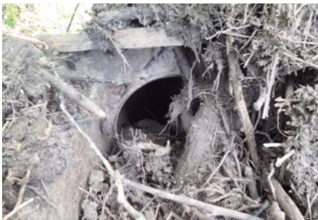
Wooded debris obstructing culvert
